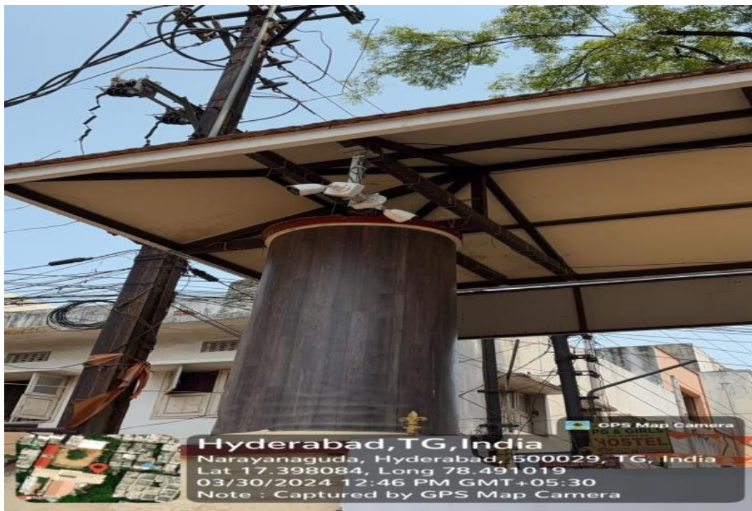
CCTV at entrance of main gate
