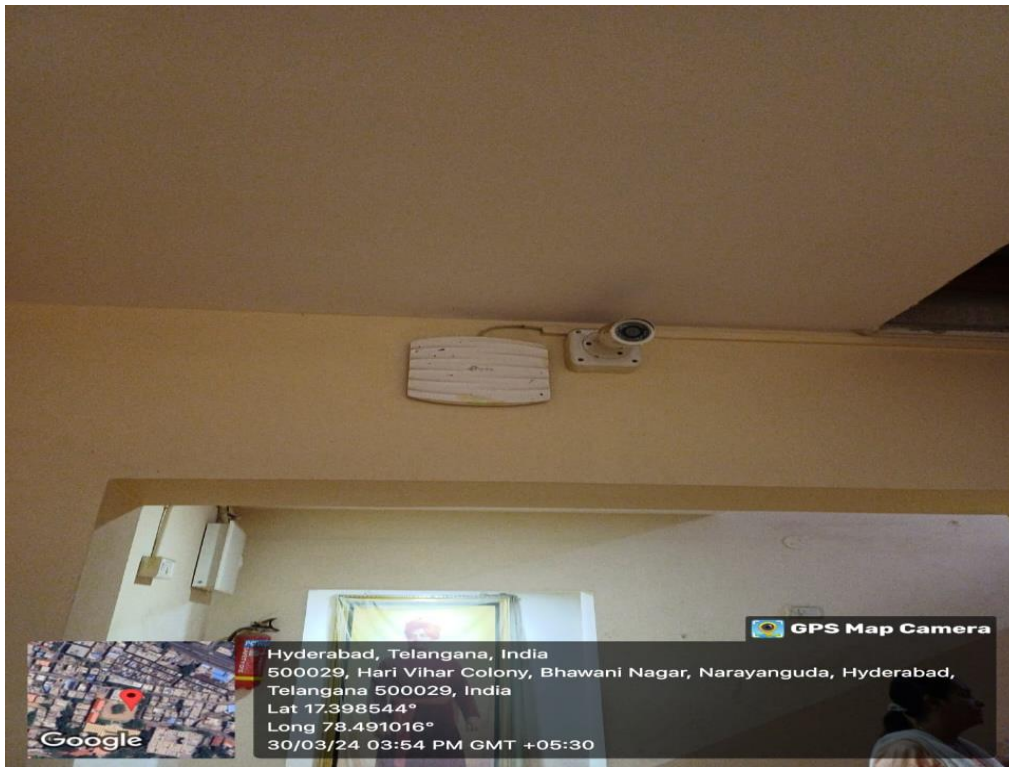
CCTV in corridors
